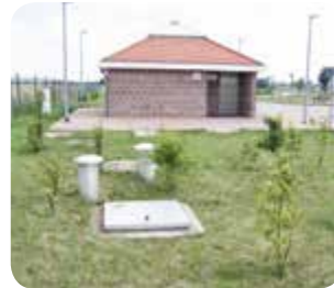
Pumping station on a motorway
